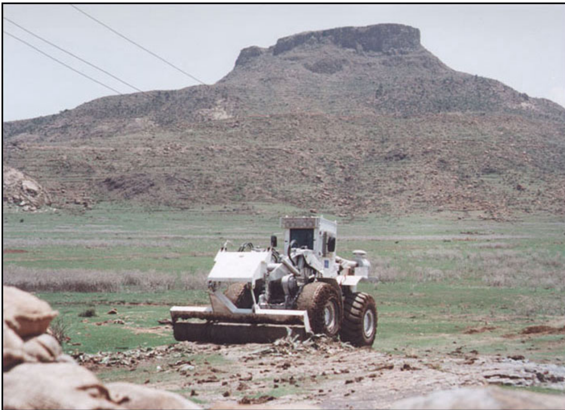
A Pearson Roller attached to a CASE front-end loader working near Senafe, Eritrea.
